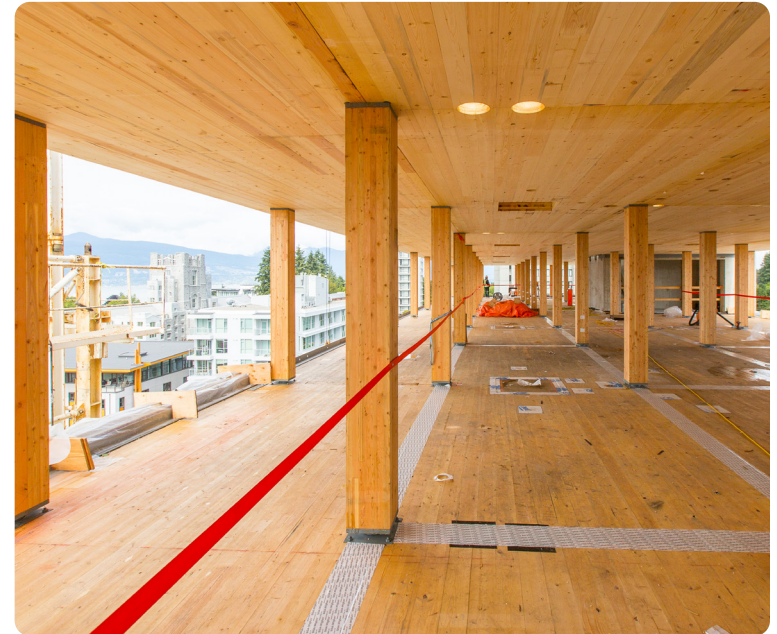
Brock Commons Tallwood House - Tall Wood Building progress. Credit: naturallywood.com Photographer: KK Law ( flickr.com )
